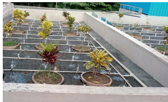
Fig. 1. Typical Soil Biotechnology Treatment plant
